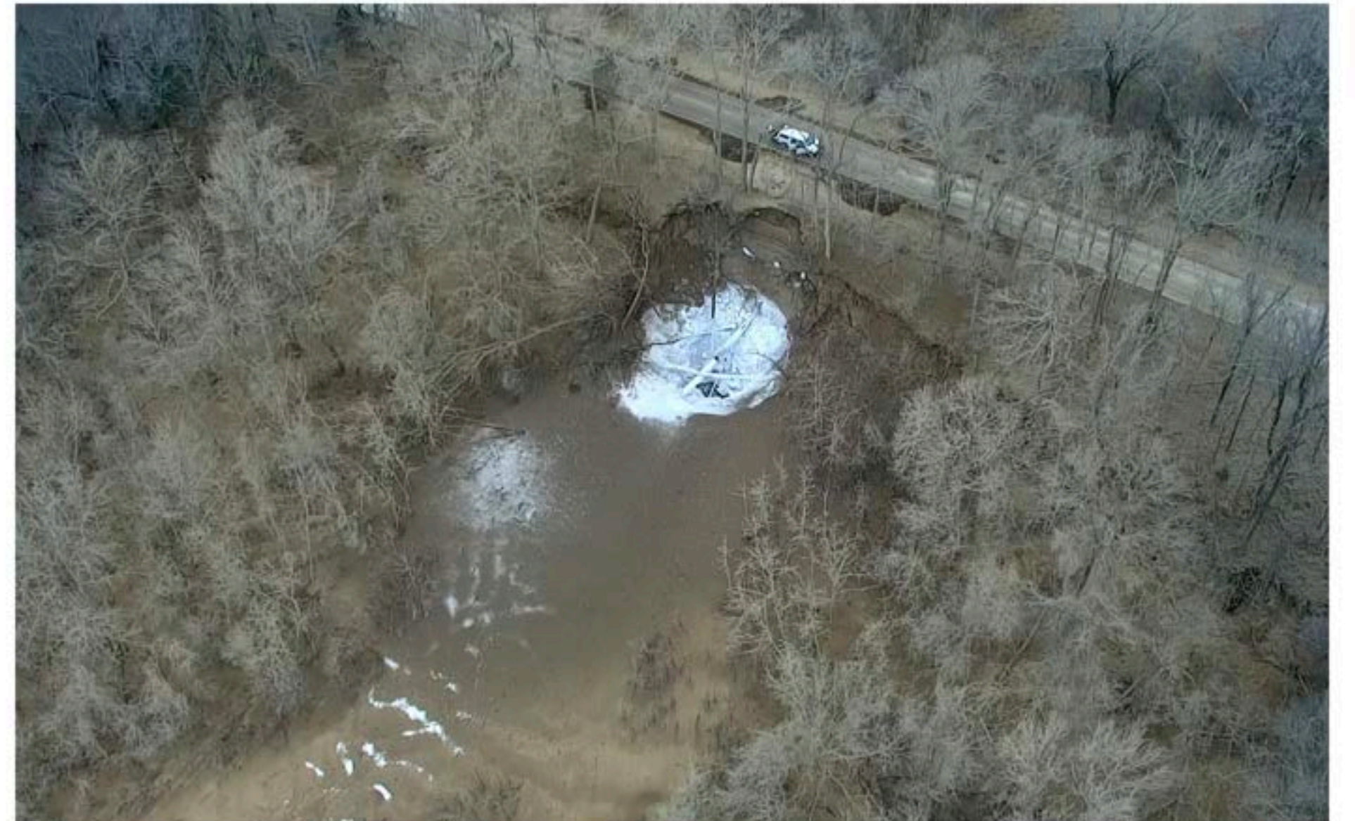
The 24-inch Denbury Gulf Coast CO2 pipeline ruptured just outside of the small village of Satartia, Mississippi, on February 22, 2020. Weeks of heavy rains resulted in a landslide that caused what the industry calls a "guillotine" failure.
